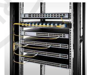
Figure 5. Switches mounted in a Rack
